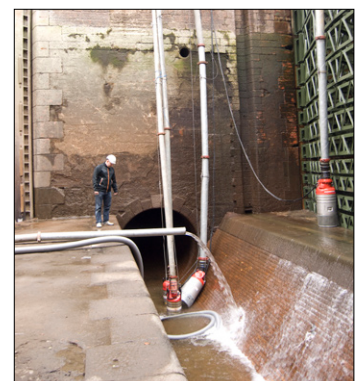
Lilla Edet, two Matador pumps drains leaking water inside of a temporary lock gate. The two Maxi pumps were used during the draining of the lock chamber.
