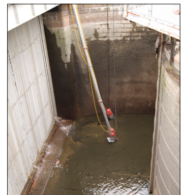
Two Matador pumps drains leaking water inside of a temporary lock gate in Lilla Edef.
