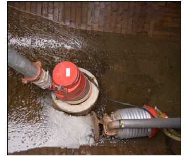
A Matador pump drains leaking water below the upper lock floor. The sludge pump Senator (laying down) is used for pumping away any fish that gets trapped in the lock.
